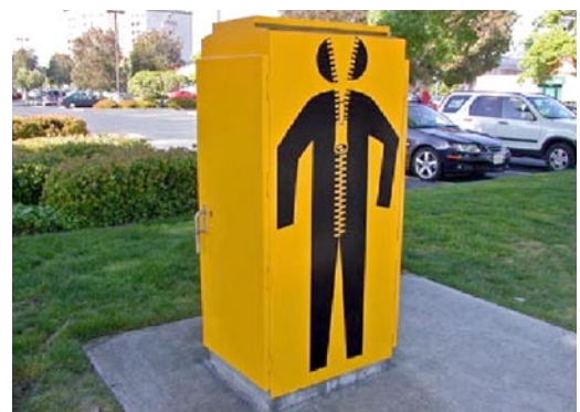
Utility box designed by Seyed and students
